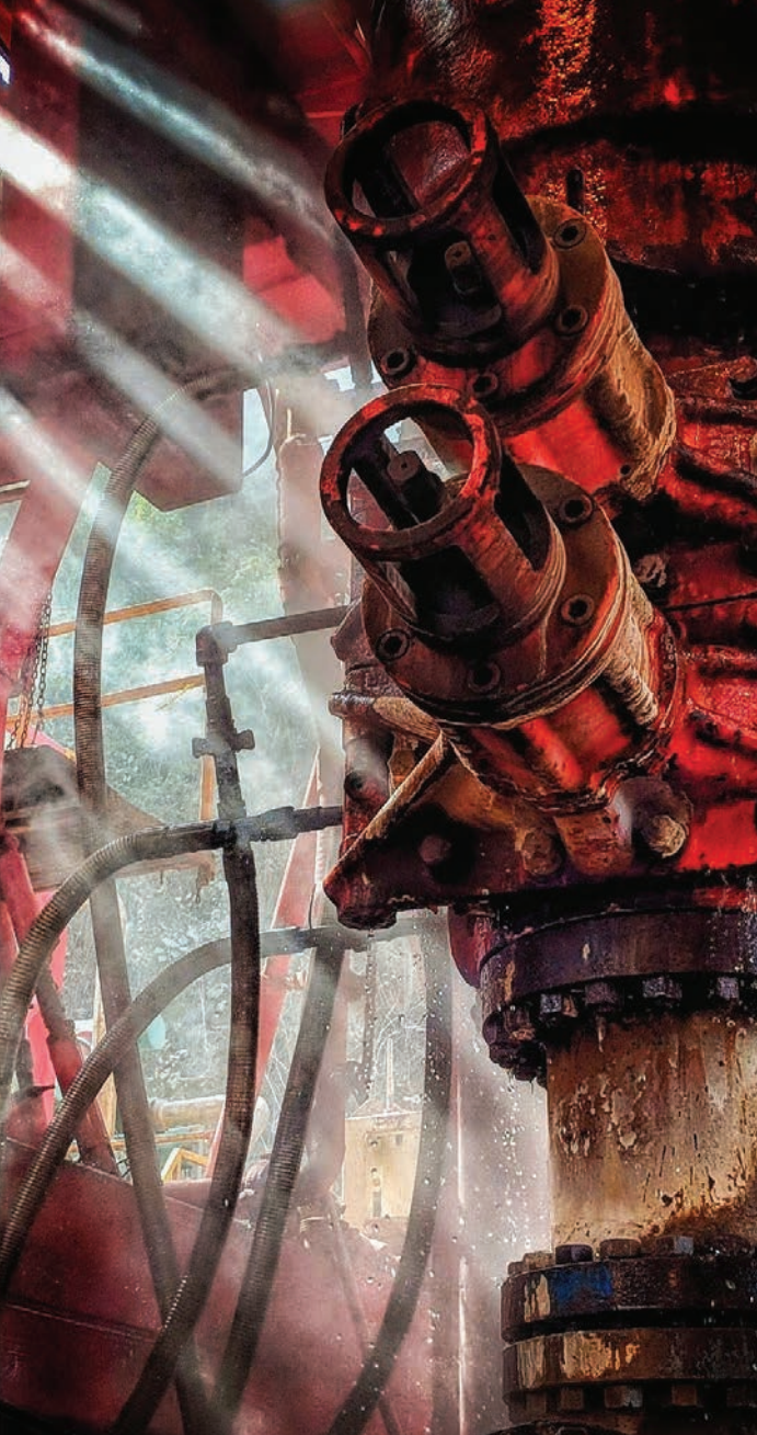
■ Reaching hot dry rock—sometimes several miles below the surface—requires complex drilling equipment and deep understanding of the Earth’s subsurface. Photo: Piyush Bakane
